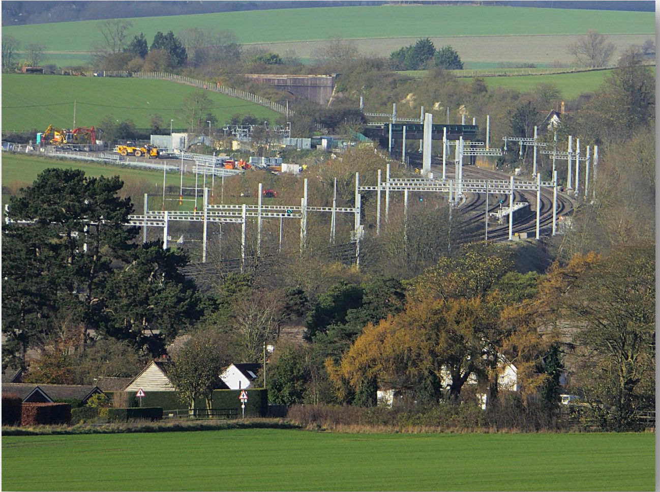
Installation of Series 1 OLE in progress in the AONBs north west of Goring (the Chilterns AONB in the foreground and North Wessex Downs in the background)
